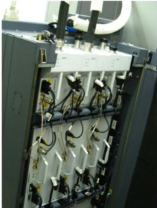
Figure 3-6: 3G Equipment Demonstration
