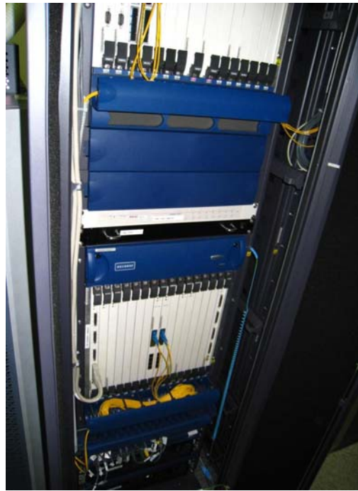
Figure 3-7: 3G Equipment Demonstration
